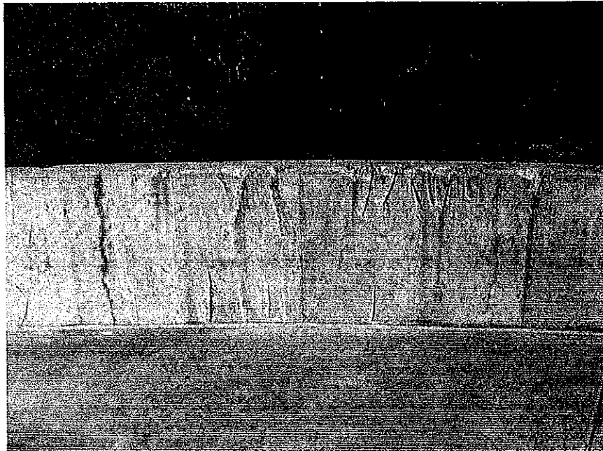
Photo 3. Minor chipping has occurred at parapet at upper level. While not a structural issue, cosmetic patches are an option.
