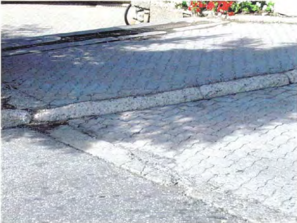
Figure 3-21a- Disrepair of concrete pavement and paverstones
