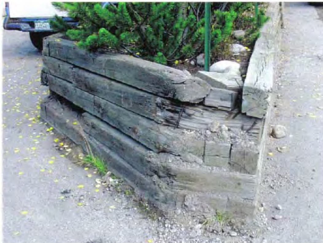
Figure 3-19a- Typical disrepair of retaining walls and planters
