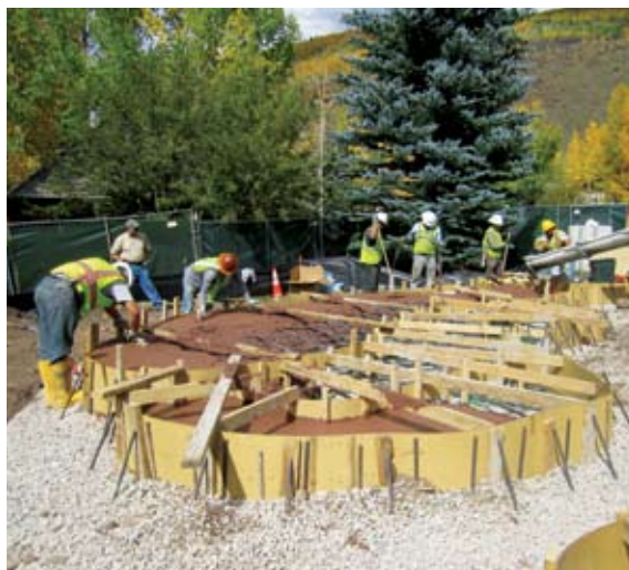
LEFT THE CREW FROM ICON, INC. OF AVON PREPARE THE BASE FOR THE AMPHITHEATER- LIKE SETTING OF THE INSTALLATION.
