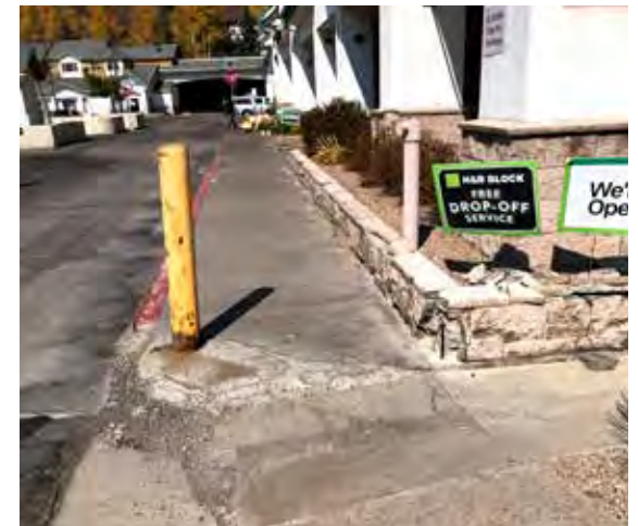
Example of a sidewalk and ramp in need of repair
