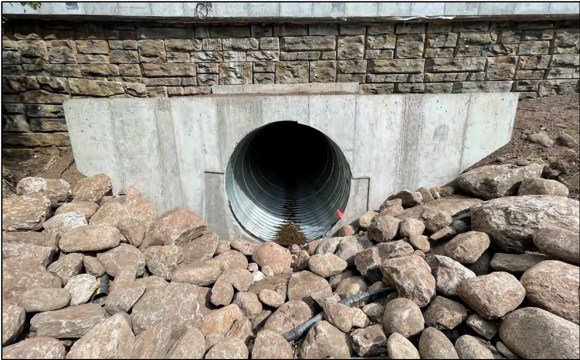
Photo 3. Recently placed cobble and new culvert at the upstream end of Middle Creek, where it flows from below the South Frontage Road. (9/28/21).
