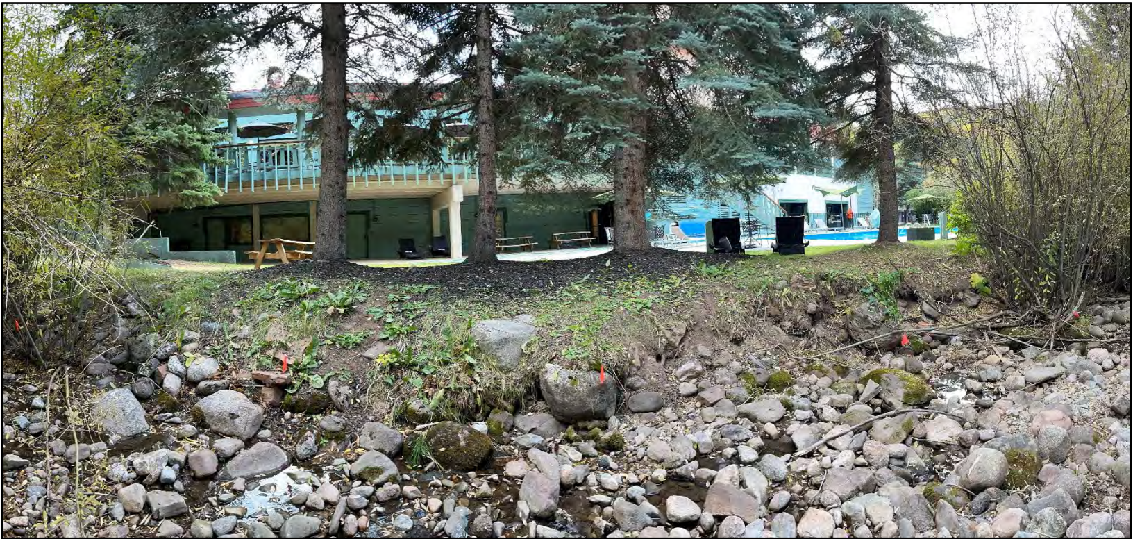
Photo 8. Eroded streambank adjacent to the Evergreen Lodge. (9/28/21).
