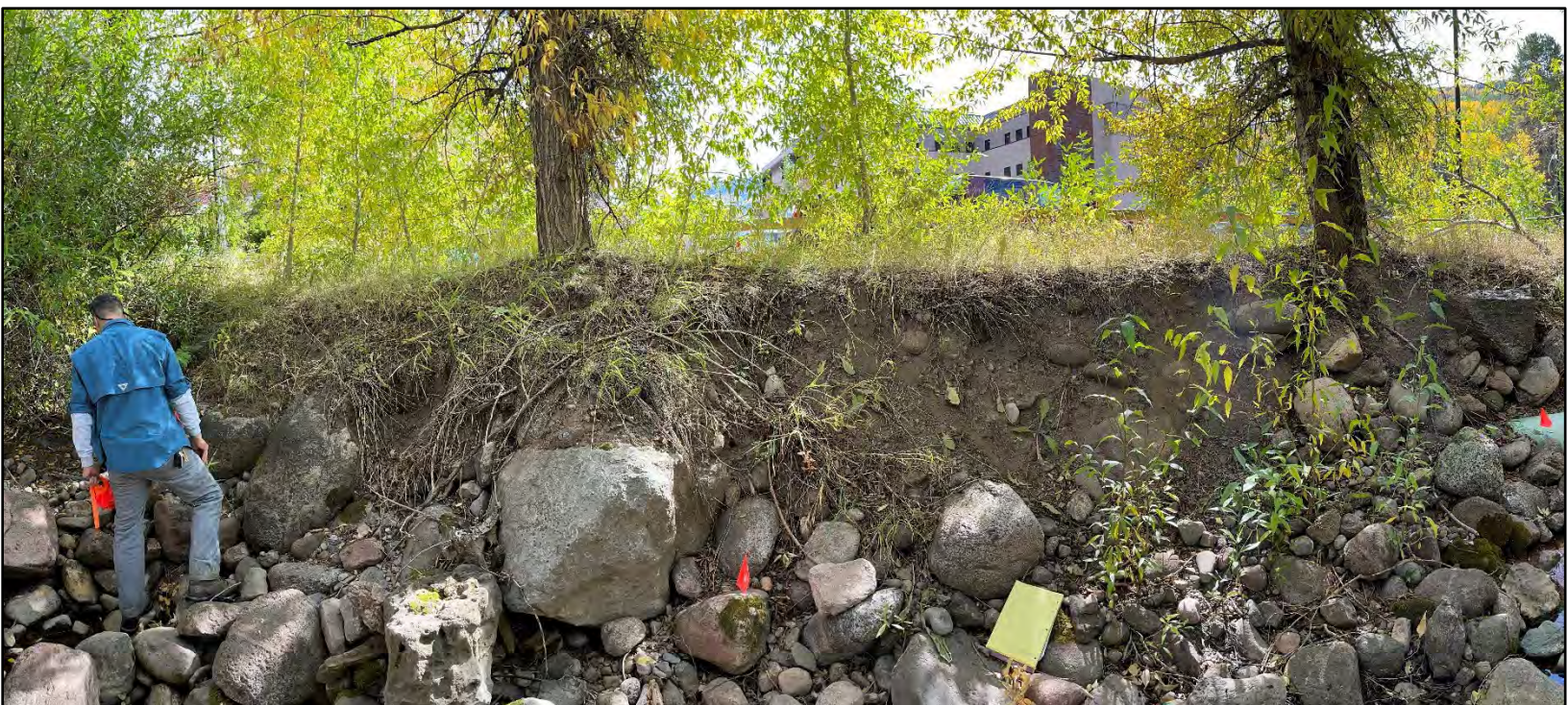
Photo 9. Steep, eroded streambank adjacent to the Evergreen Lodge. (12/7/21).
