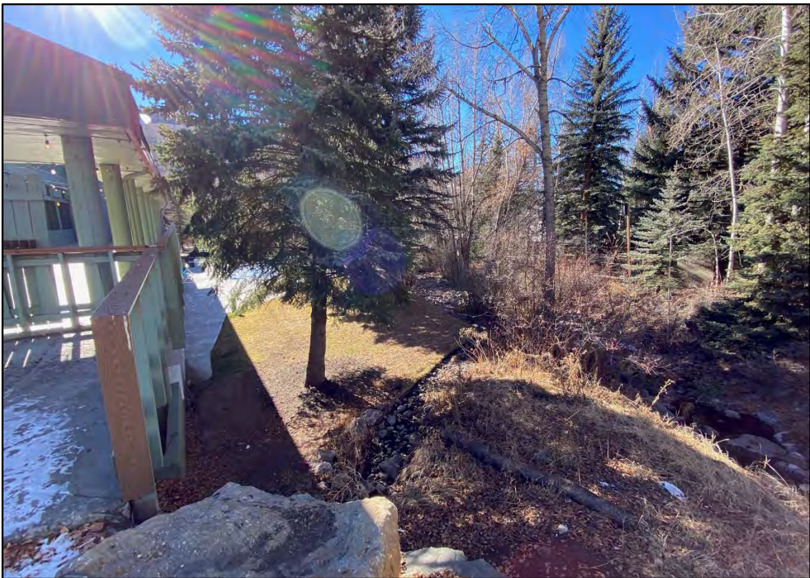
Photo 12. Saturated soils occur within a small, constructed swale extending from the foundation dewatering system to the creek. (12/7/21).
