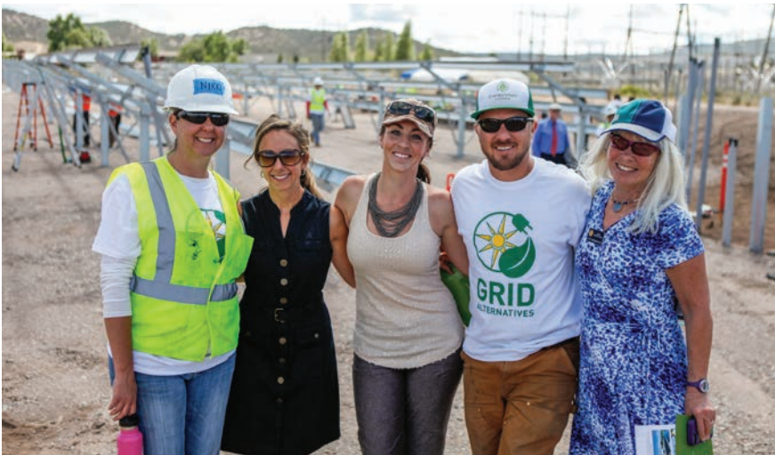
Holy Cross Energy board members and community volunteers installed a new solar array in Gypsum.
