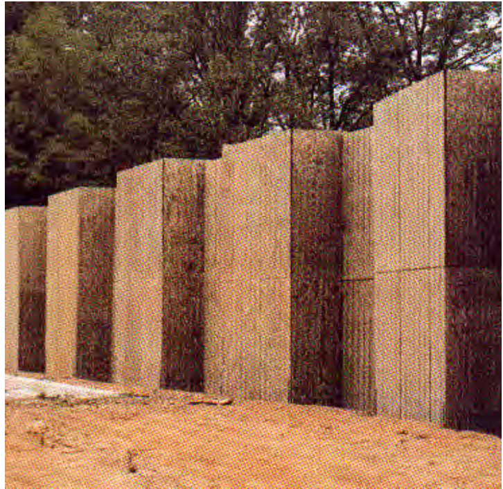
Plywood Noise Wall
