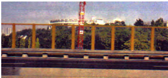
Glass Noise Wall, France
