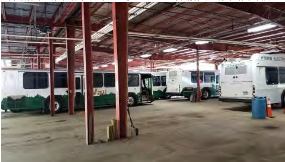
Bus storage area LED lighting with motion sensor control.
