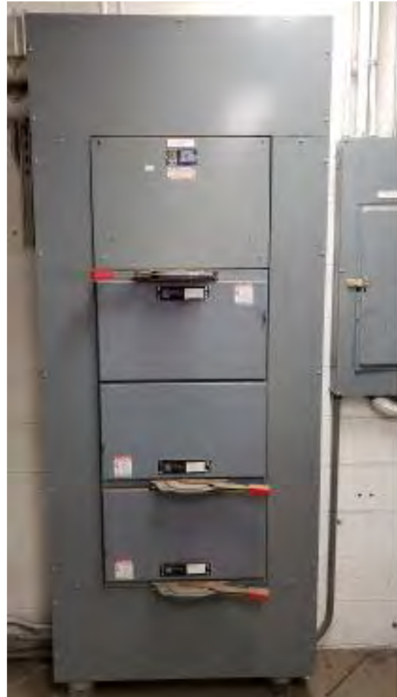
Maintenance Building Main Distribution Panel, one of two.
