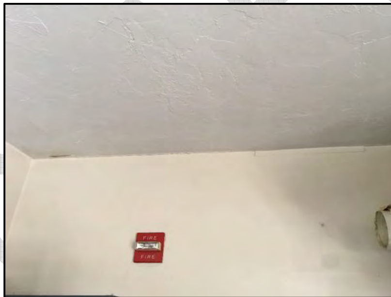
Photo 10: Crack Between Ceiling and Wall in Mezzanine Office
