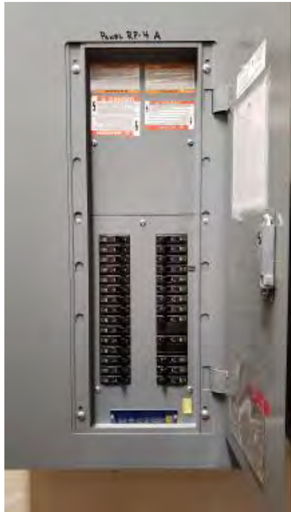
Administration Building Main Power Panel.
