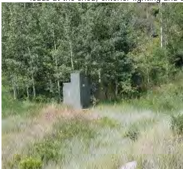
Utility transformers at northwest corner of property. These feed the Admin building and housing.
