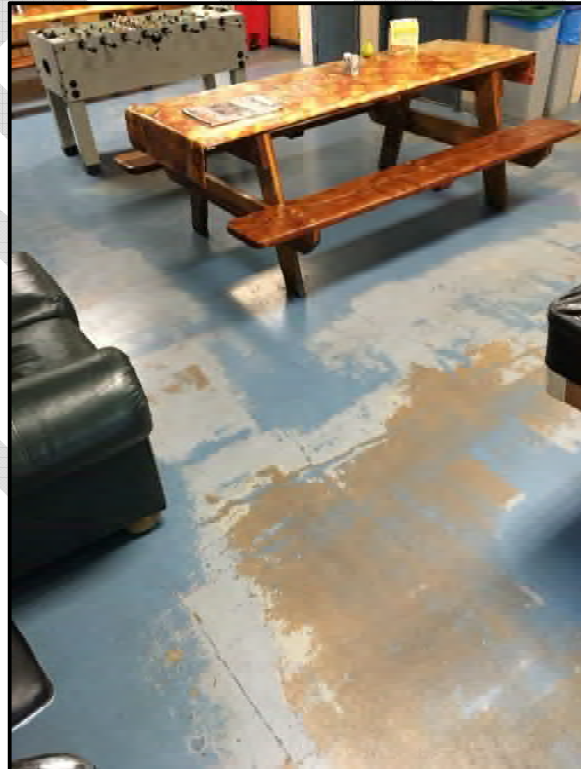
Photo 8: Cracking in Mezzanine Slab on Metal Deck at Break Room
