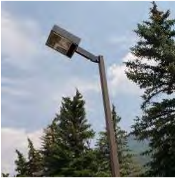
Pole mounted LED fixtures at Site
