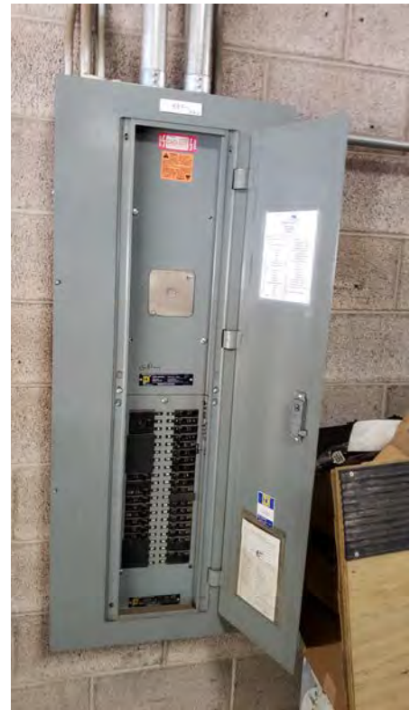
Maintenance Building typical power panel
