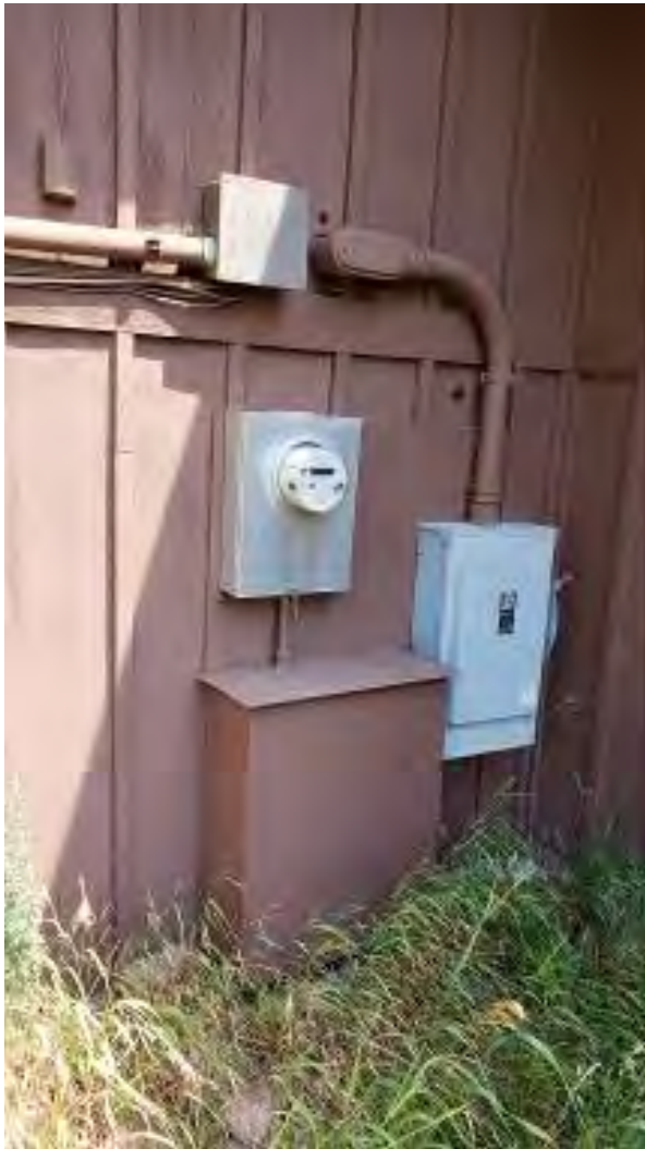
Administration Building incoming service CTs and Main Disconnect
