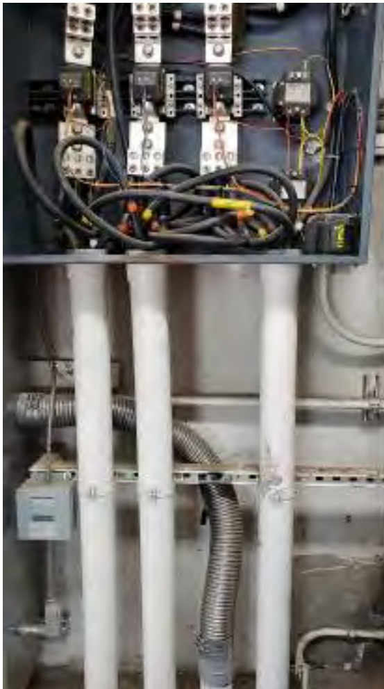
Maintenance Building incoming service splice at CTs
