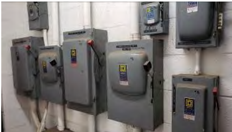
Maintenance Building old gutter and disconnects
