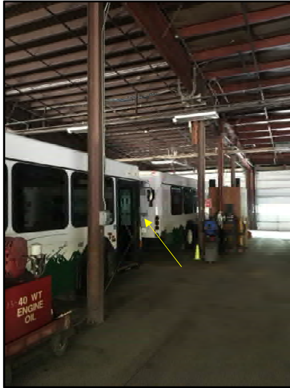
Photo 3: Tension Only Steel Cross Brace Missing Tension Tie
