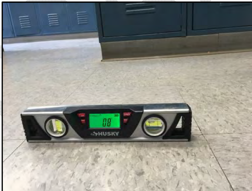
Photo 6: Hump in Mezzanine Locker Room
